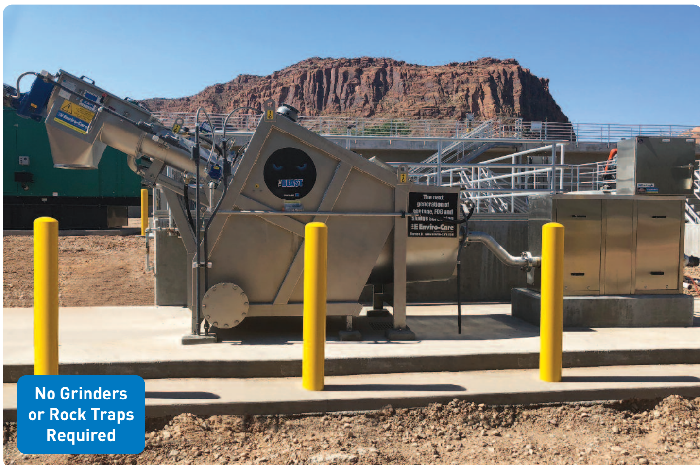
Septage BEAST Property of Moab UT
