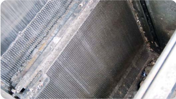
Perforated media attached to dead plate.
