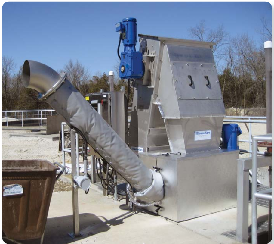
Flo-MultiRake screen and Flo-WashPress installed at the Cuba MO WWTP headworks
