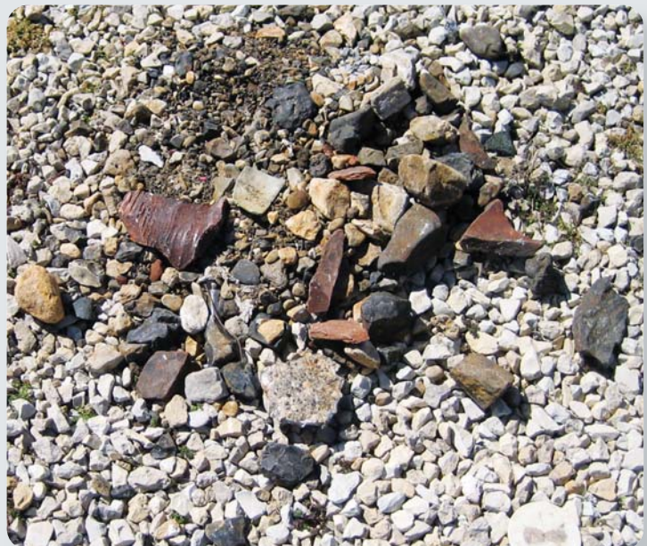
Pieces of clay tile and large debris washed to the headworks during heavy rains.
