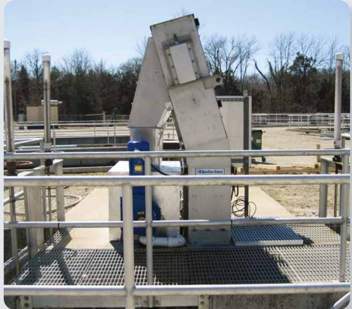
Flo-MultiRake Fine Bar Screen with 6 mm bar spacing installed at a 90° angle.
