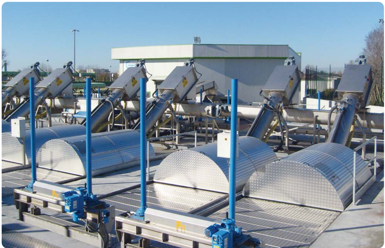
Six FD-MBR2000 10 MGD Per Screen - Brescia Italy
