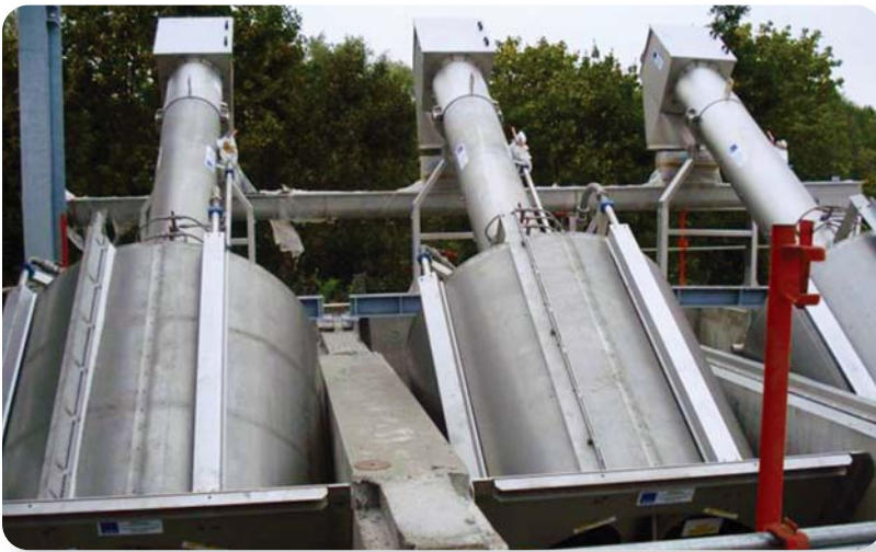
Three - FD-MBR2000 5 MGD Per Screen - Orleans, France
