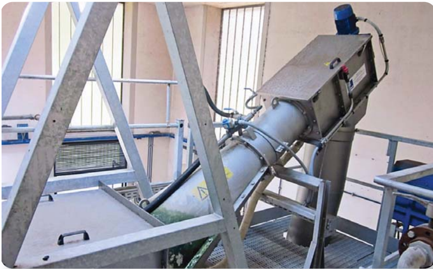
A Flo-Sieve unit installed at a 2 mgd plant.
