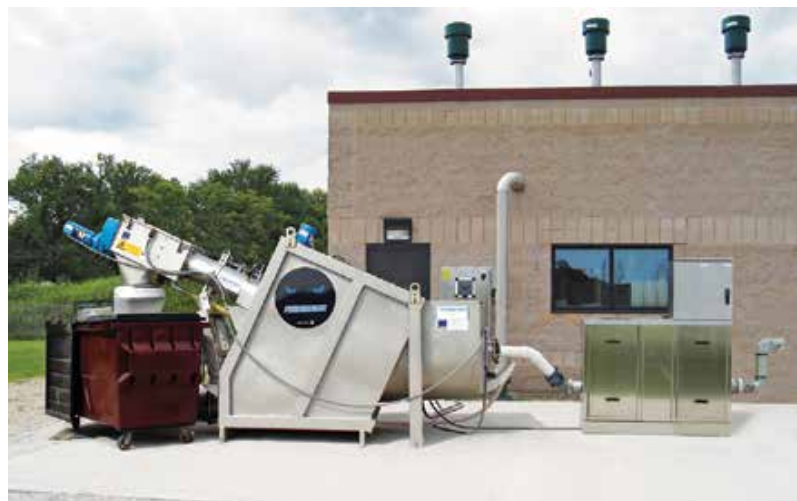
The Beast septage receiving system (Enviro-Care) at Richmond includes a screen, hauler station, and hauler access panel.
