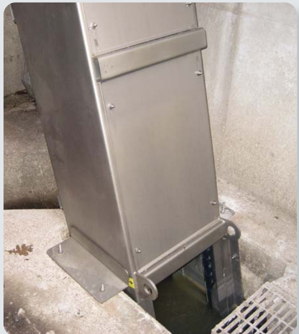
A turnkey, "plug and go" retrofit.
