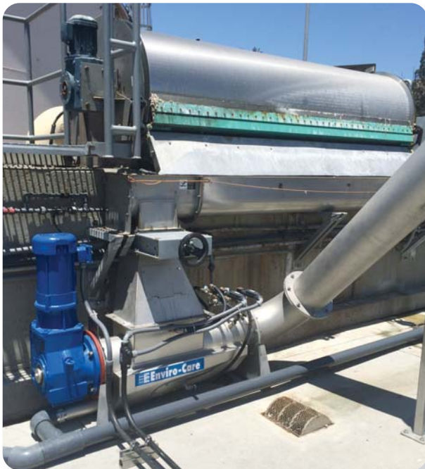
A SAVI® VWP-2 Washer Compactor receiving screenings from a launder system.
